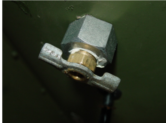
Drain Fitting Open
